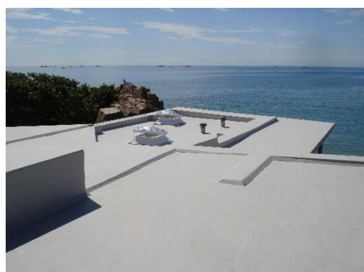
Long-term protection: Coastal Installations
